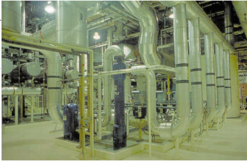
Piping feeds and filter unit at the WCM
